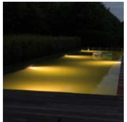
LED recessed floodlights.
